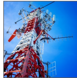
Telecommunication Base Station
