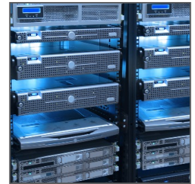
Rack Mount Server
